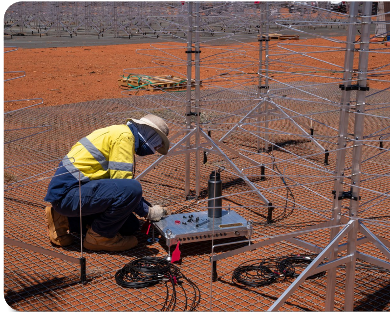
ABOVE: SKA-Low Field Technicians will install 24 SMART boxes per station.
